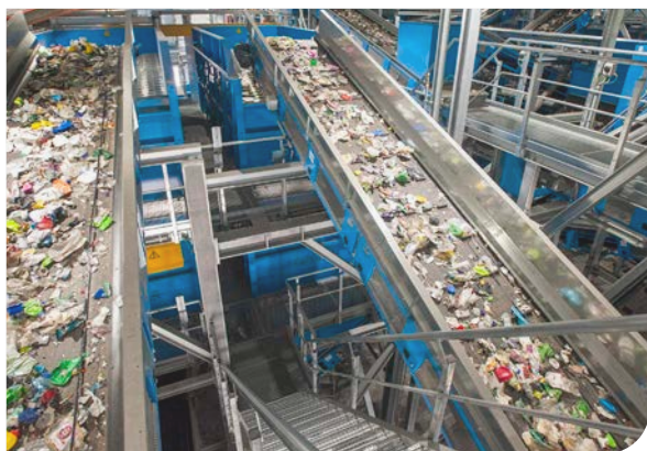
Viridor Materials Recycling Facility separating co-mingled recycling
